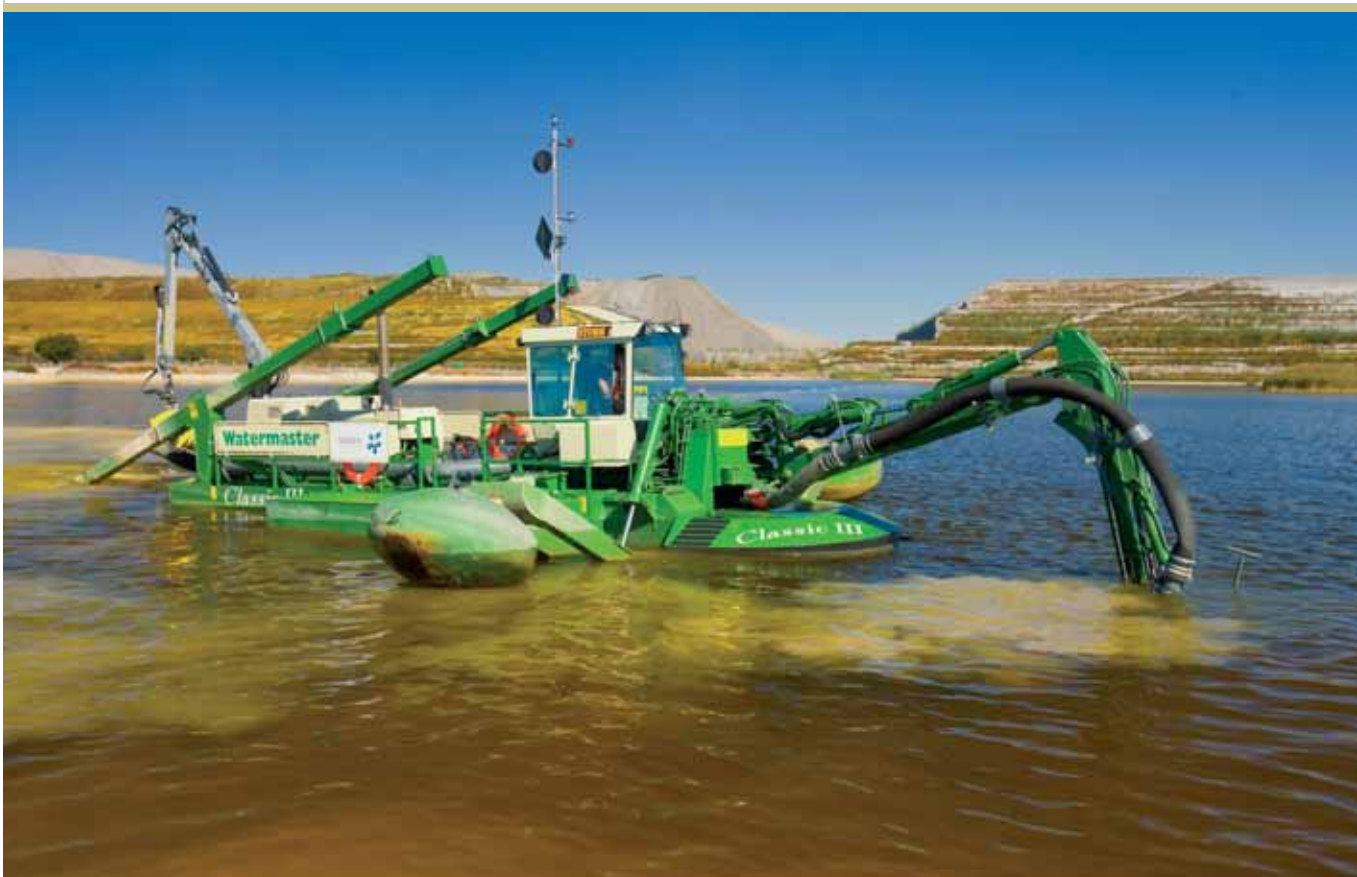
A dredger removing sediment from an evaporator dam to increase capacity for water received from Secunda plants, as well as rain water.
