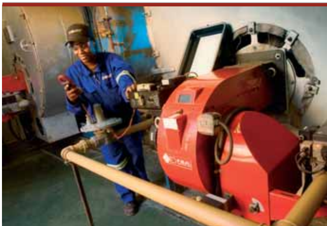
Gas boiler operation at Isover, a manufacturer of insulation fibreglass.
